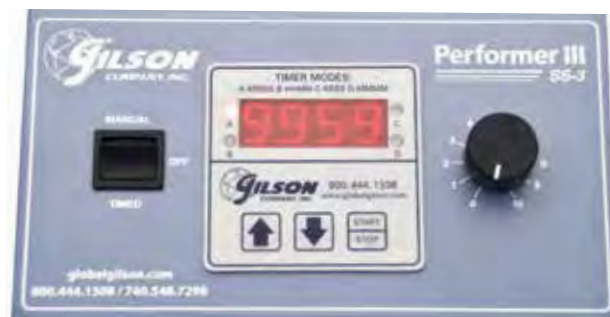
SS-3 control panel
