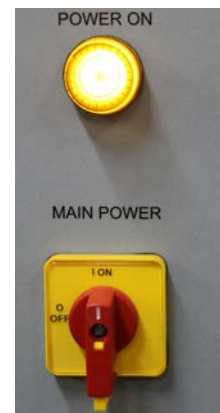
Figure D.2 - Power switch in the ON position
