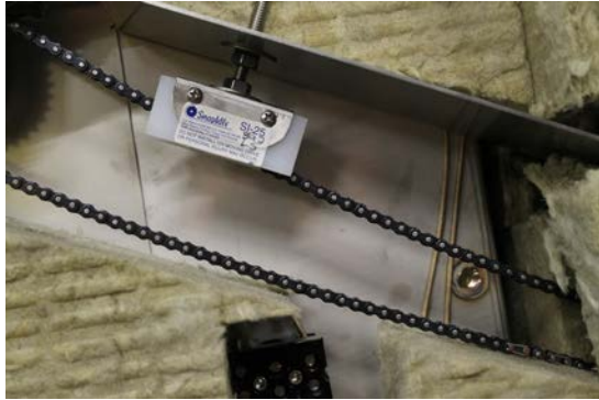
Figure H.9: Chain is too loose
