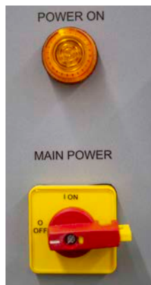
Figure D.1 - Power switch in the OFF position
