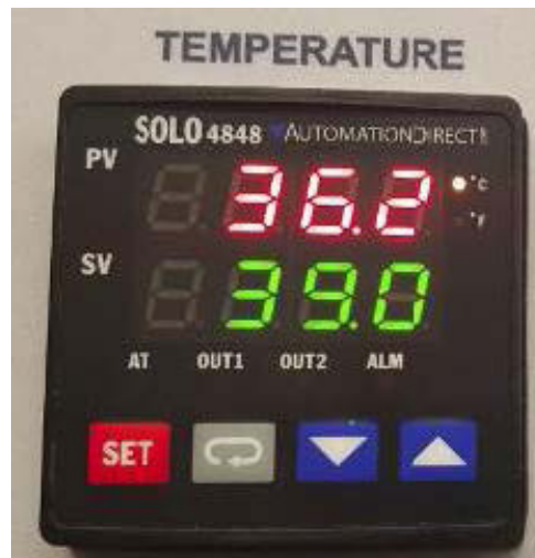
Figure D.6 - Temperature Controller
