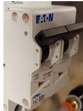
Figure G.2: Circuit breaker in the ON position
